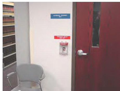
Fire Alarm in Law Library
